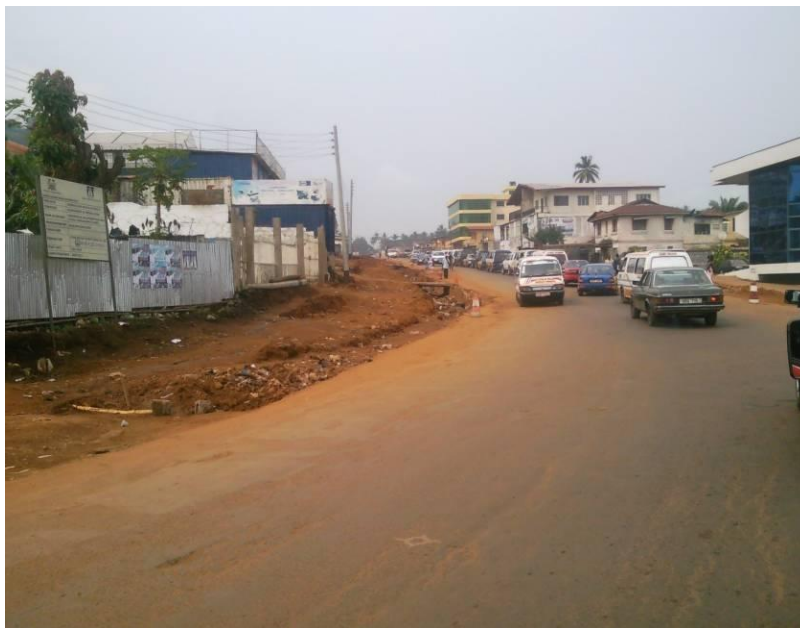
Wilkinson Road, Freetown. The road is being widened into a Dual Carriageway. It has implications for Road safety
